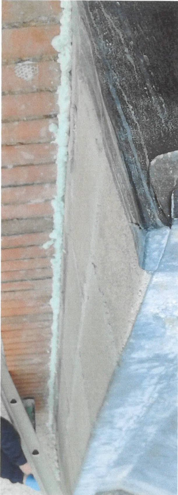
Outer leaf of blockwork forming parapet. Note foam filled gap between new extension walls and existing party/party wall.
