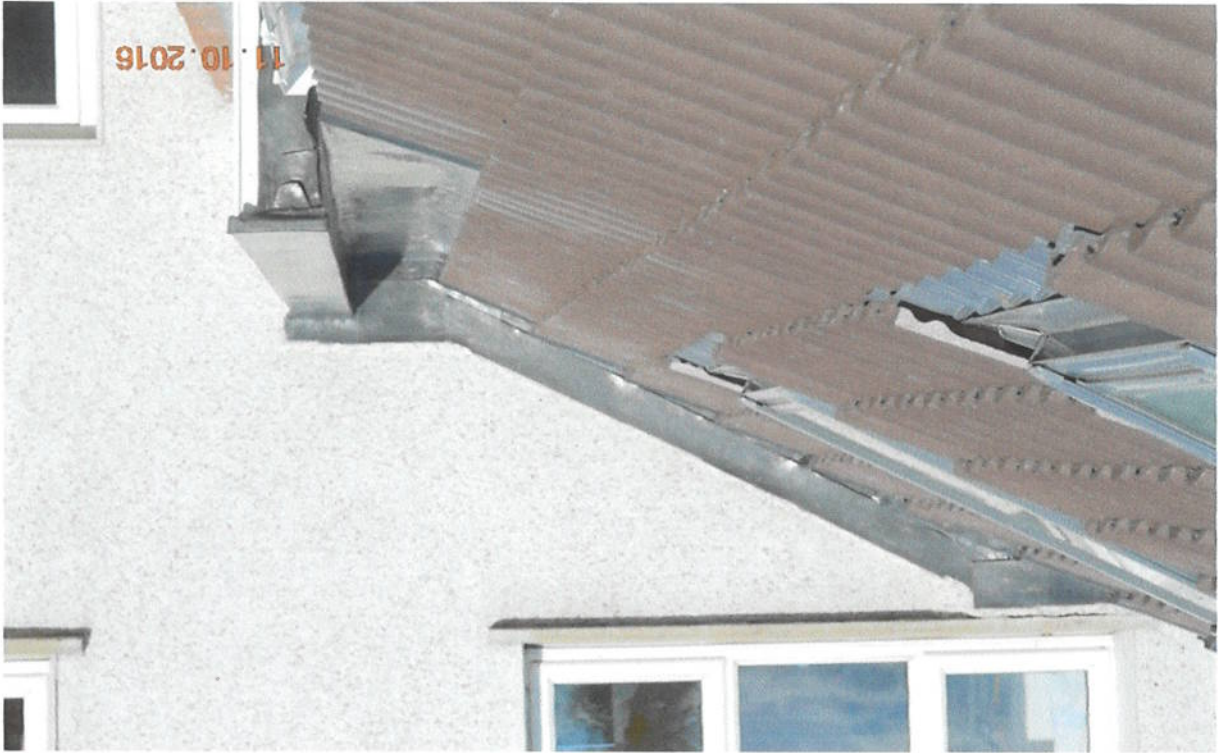
The picture above clearly shows the outer leaf of blockwork forming the parapet detail. Note the existing red brick capped party/party wall.
